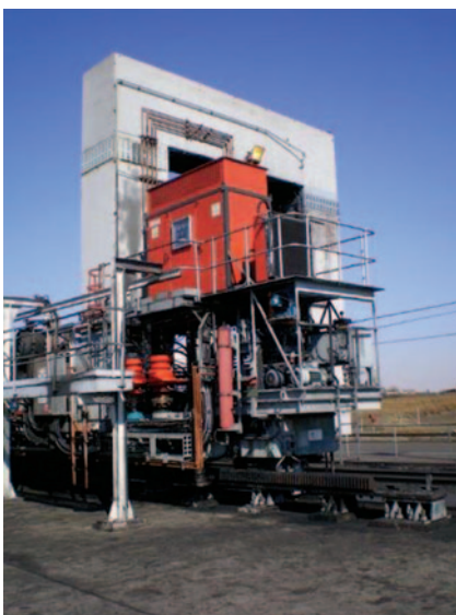
DemcoTECH's recommendation for upgrading and enhancing of the coal off-loading and delivery system for a South African power utility included the tandem wagon tippler.
