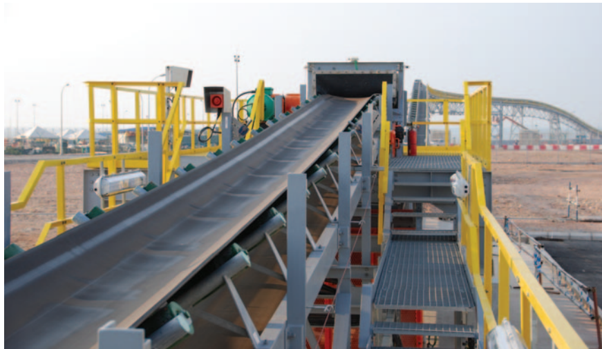
Turnkey Petronas RAPID project in Malaysia.
