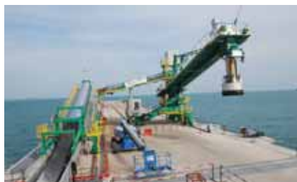
RAPID project: shiploader with telescopic chute minimizes dust generation.
