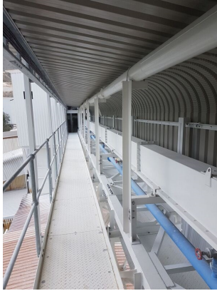
Air slide on gantry – part of the DemcoTECH-designed discharge materials handling system for the newly installed Loesche Mill Plant at Idwala Carbonates.
