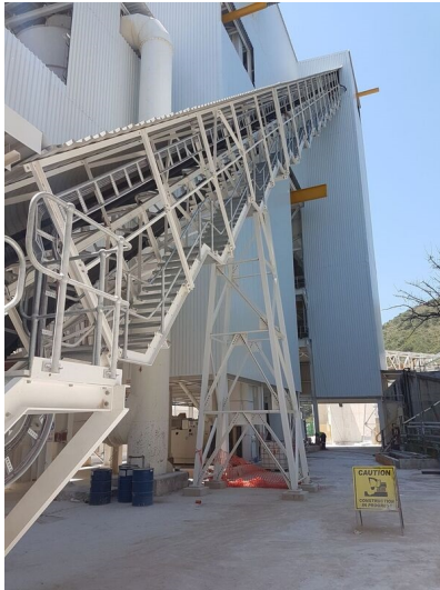
Pocket conveyor 40 degree incline gantries - part of the DemcoTECH-designed feed materials handling system for the newly installed Loesche Mill Plant at Idwala Carbonates.
