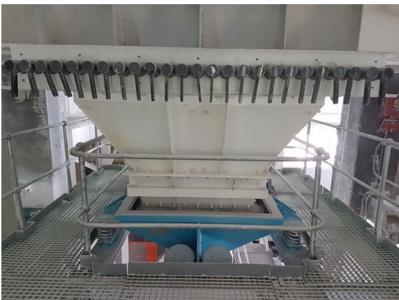
Existing bin modification with rod gate and vibratory feeder - part of the DemcoTECH-designed feed materials handling system for the newly installed Loesche Mill Plant at Idwala Carbonates.
