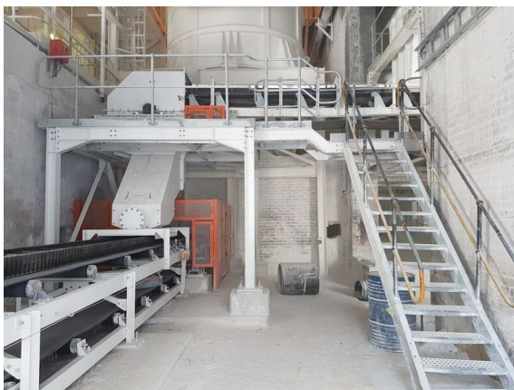
750 mm wide belt conveyor - part of the DemcoTECH-designed feed materials handling system for the newly installed Loesche Mill Plant at Idwala Carbonates.
