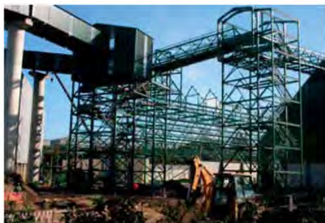
Construction of conveyors and transfer house at the Richards Bay multi-product terminal, KwaZulu-Natal, South Africa.
